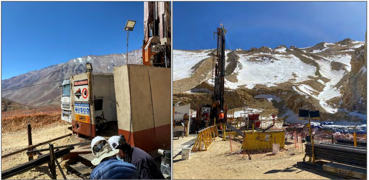
Figure 9-3: Drill sites in operation during Phase II (left) and Phase III (right).
